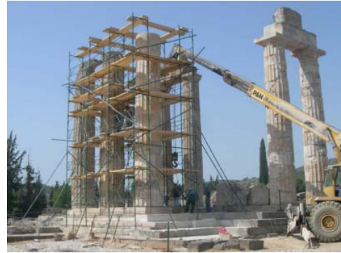
Crane donated by Titan in use erecting column. (Source: Makris Report on Reconstruction 2007)
