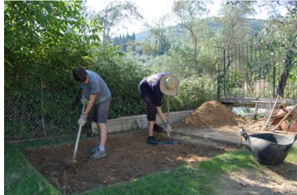
Students Ryan Boehm and Doug Parada excavate area for a new restroom for guards at the Museum.
