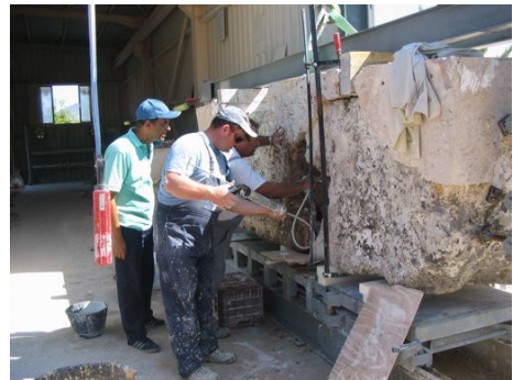
Our Consulting Engineer, Dr. Kostas Papantonopoulos, and two of our excellent workmen, Christos and Elias, work on restoring an epistyle.
